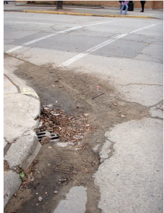
Figure 6.2. Sediment clogging a storm drain adjacent to a construction site in the Monona Bay watershed.
