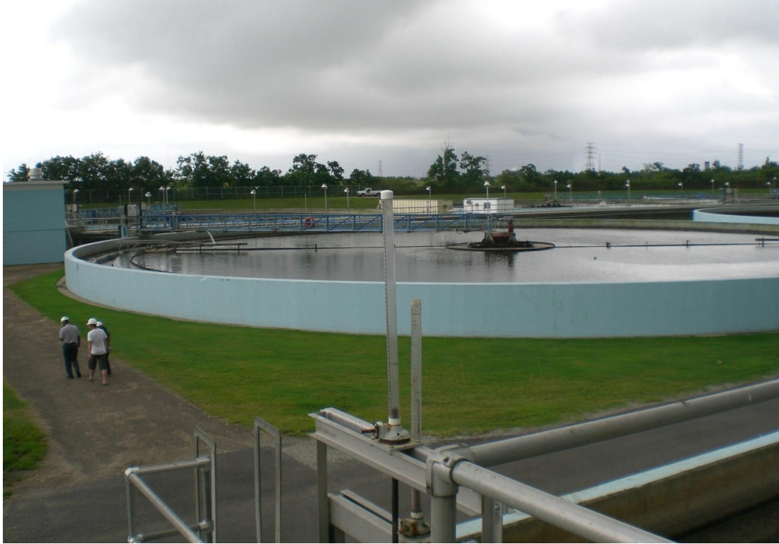
Figure 4-5: One of eight clarifiers at the EBWTP. (Photo by Dan Cornelius, July 2008)
