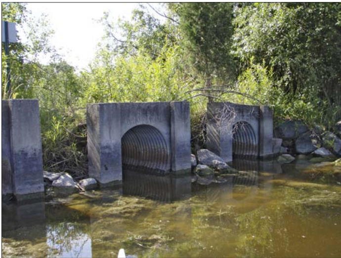
Figure 3.12: Erosion of earthen berm supporting the CCC Dam control structure.
