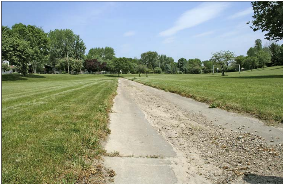
Figure 7.1: Existing conveyance channel in the Arbor Hills Greenway. Visible are large amounts of sediment and particles transferred from the upstream watershed to the Eastern Marshes.
