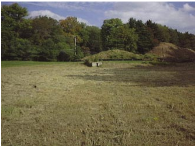
Figure A10-1. An existing stormwater detention basin was targeted for a CWA 319 retrofit project.
