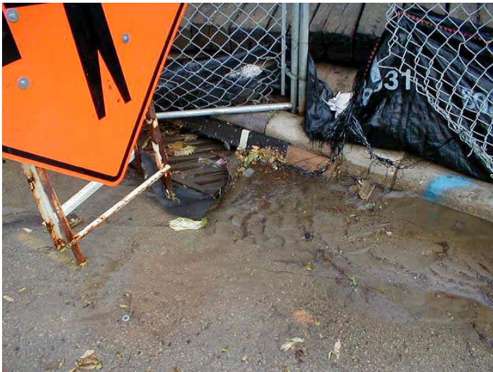
Figure 4.2. Poorly maintained inlet protection and defective silt fence near Chamberlin Hall.
