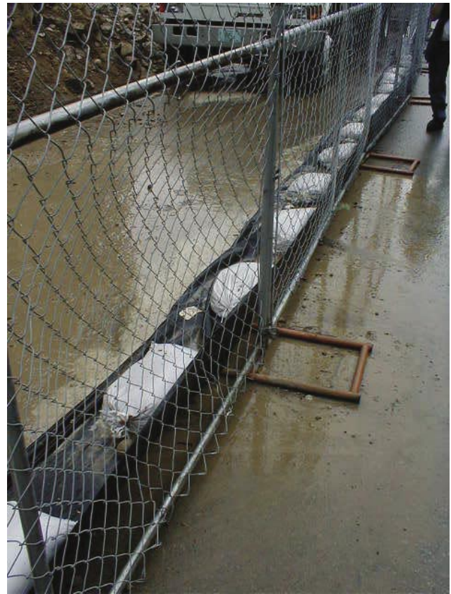
Figure 4.1. Ineffective silt fence near Chamberlin Hall.
