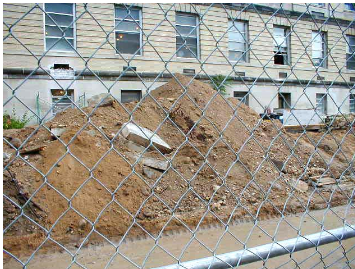
Figure 4.5. Large uncovered dirt pile near Chamberlin Hall.
